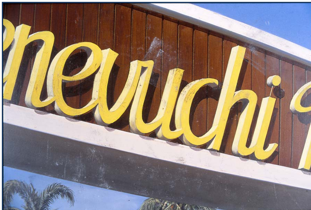
MGM 154 - Detail - Surface cleaning needed
